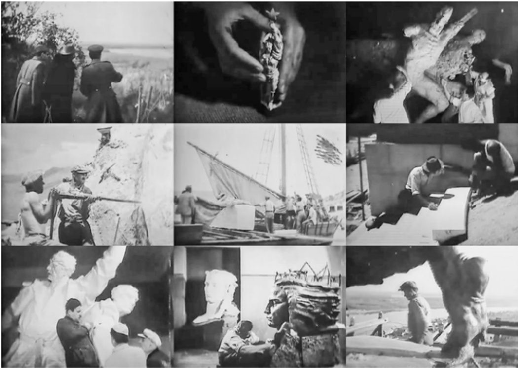
435 Frames from the film Monument in Gratitude to the Red Army (director Milan Katić, 1948), showing different phases of the construction of the monument in Batina, Croatia. For images of the monument, see figs. 118–122.
